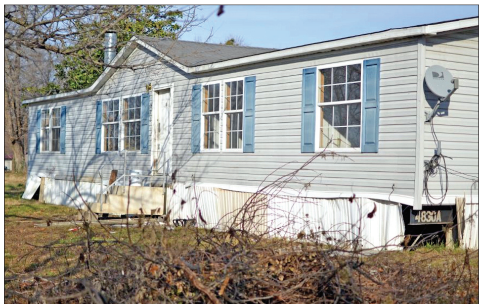
Extensive skirting damage on mobile homes can be a welcome mat for wildlife seeking shelter from the cold during the winter months.
